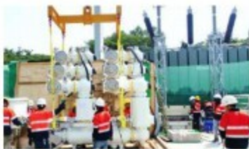
Our GIS Installation Engineer of Myanmar for M/s. GE Global Operation.
