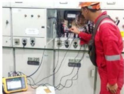
Harmonics Measurement at M/s. Power Engineering and Technology in Cilegon, Indonesia
